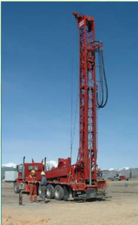
PRE-DRILL AIR UNIT
