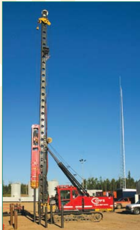
TRACK MOUNTED UNIT
